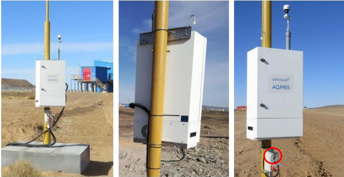
Figure 3 The AQM 65 is mounted to a pole, an additional power point is added to allow a laptop or Aircal 1000 calibrator to be plugged in.
