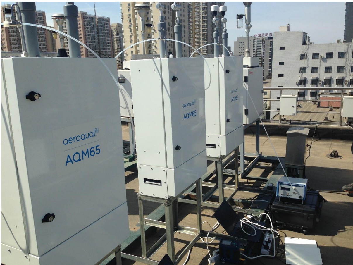
Figure 5-4 The Ozone calibrator and AirCal 1000 can calibrate multiple instruments at the same time.
