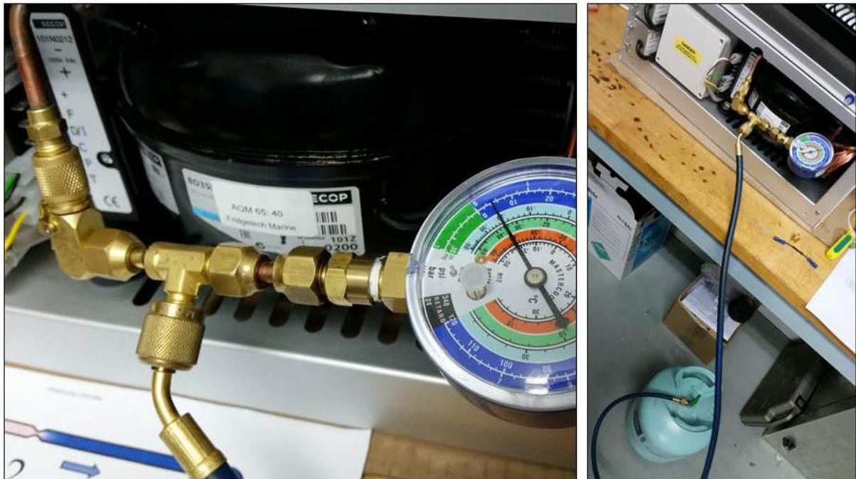
Figure 4-38 Hose attached to the pressure gauge and to the cylinder of R134a
