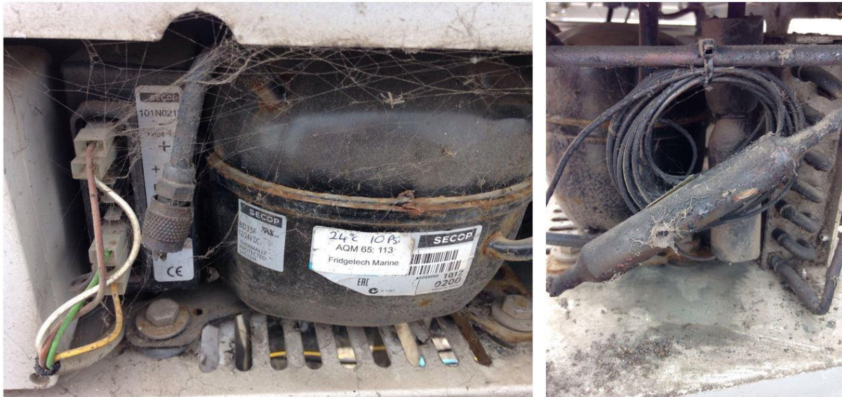
Figure 4-29 Dirt and debris can accumulate within the TMS cassette leading to reduced efficiency of the thermal management system.
