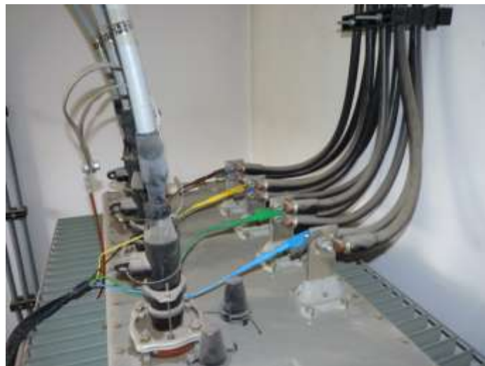
Figure 8 Connection to LV terminals on a distribution transformer
