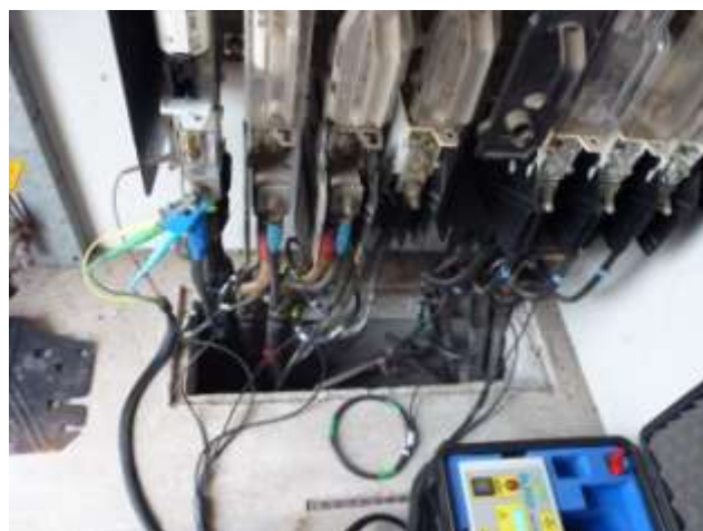
Figure 9 Installation of current coils on each feeder in a TUR type substation
