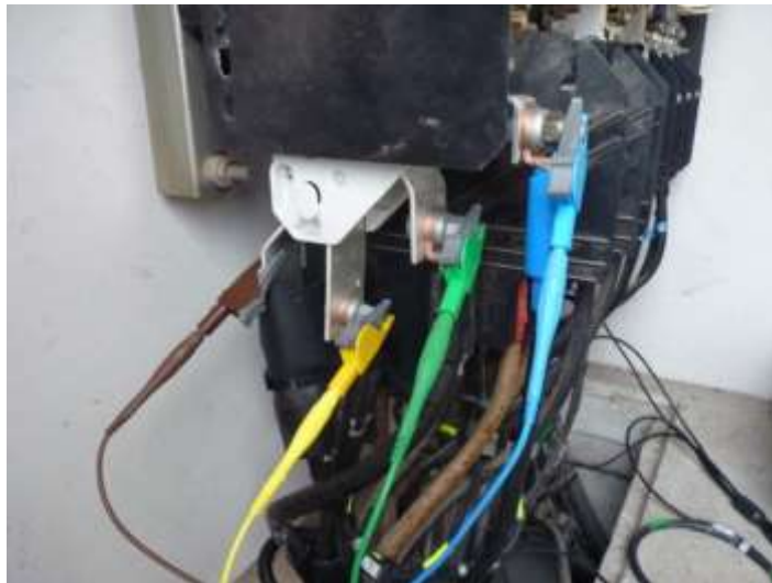
Figure 7 Voltage connections by croc clips on a feeder in a TUR type substation
